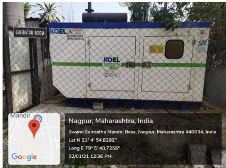
Diesel Generator in college
