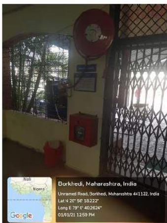
Fire Extinguisher system in college
