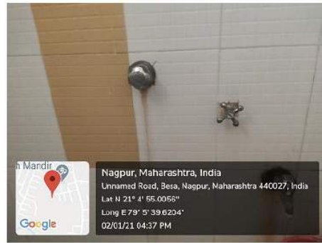
Flush to be replaced by push buttons
