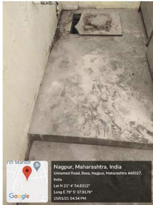
Tank constructed in college to accumulate rain water
