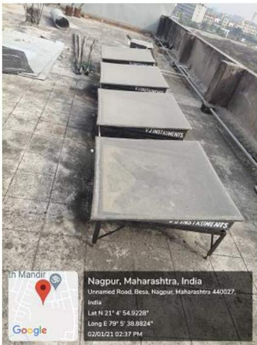
Solar Pv System for Water Distillation System
