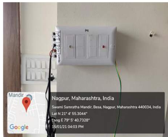
Sensor based lighting installed in college
