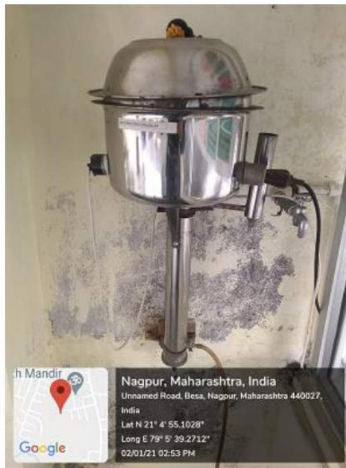
Water Distillation System operated by Solar Energy
