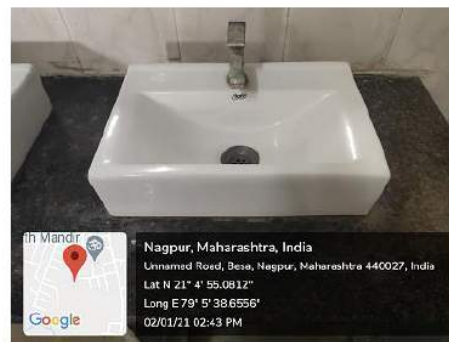
Taps to be replaced by faucets
