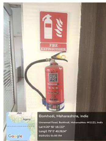
Fire Extinguishers in college
