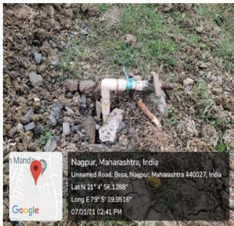
Bore well only source of water
