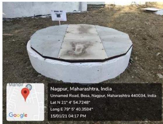
Soak pit to recharge harvested rain water to ground
