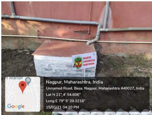
Liquid waste collection tank
