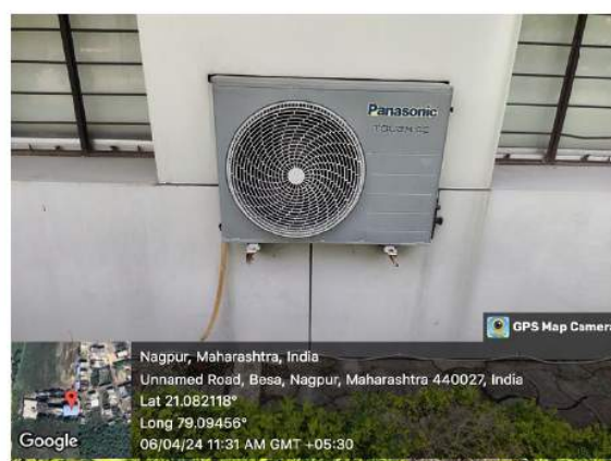
AC condenser in shade
