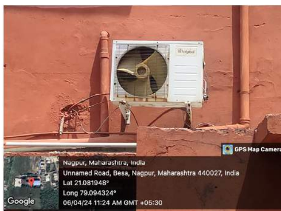
AC condenser Exposed to direct sunlight
