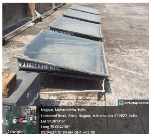
Solar Pv System for Water Distillation System
